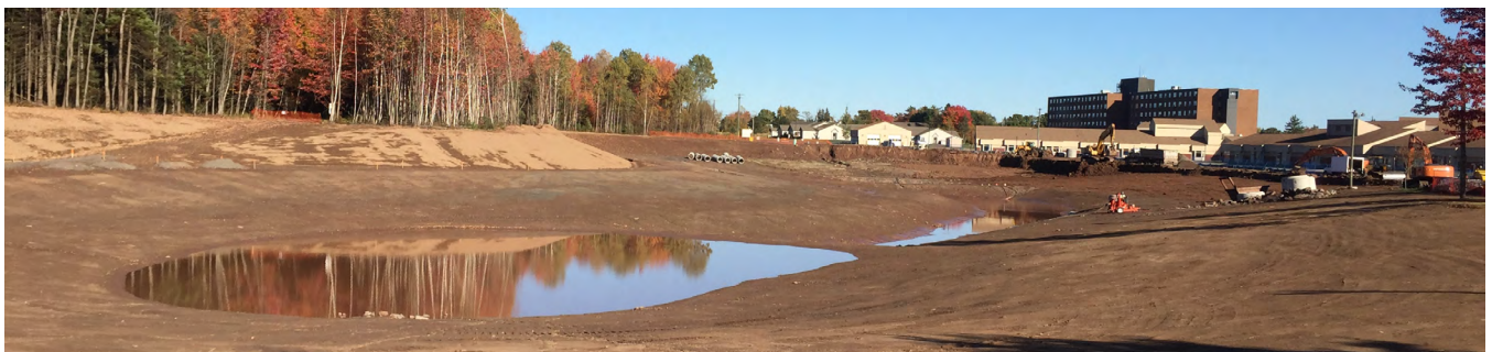
A naturalized stormwater retention pond (City of Moncton) that can evolve to provide natural infrastructure benefits. Photo ©Ducks Unlimited Canada. Used with permission.
